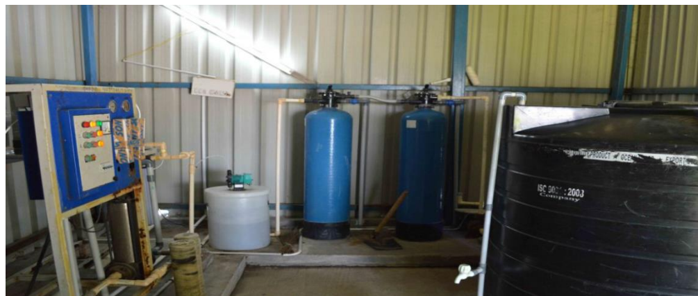
Reverse Osmosis Plant - AAACET
